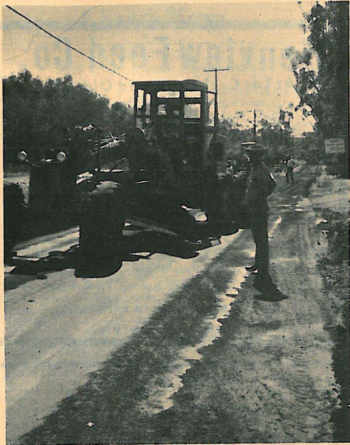
BLACKTOP IS SPREAD ON TAVERN ROAD MONDAY. THE CREWS HOPE TO HAVE JOB COMPLETED BY WEDNESDAY. (Staff Photo)
